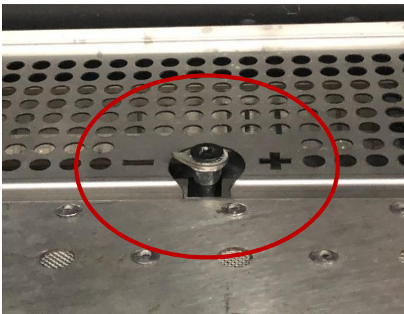
EX 1: AIR SHUTTER ON INSIDE OF FIREPLACE ON THE BURNER
