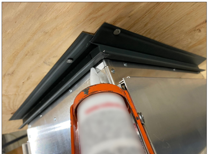
Figure 2.9, Silicone Finishing Materials
