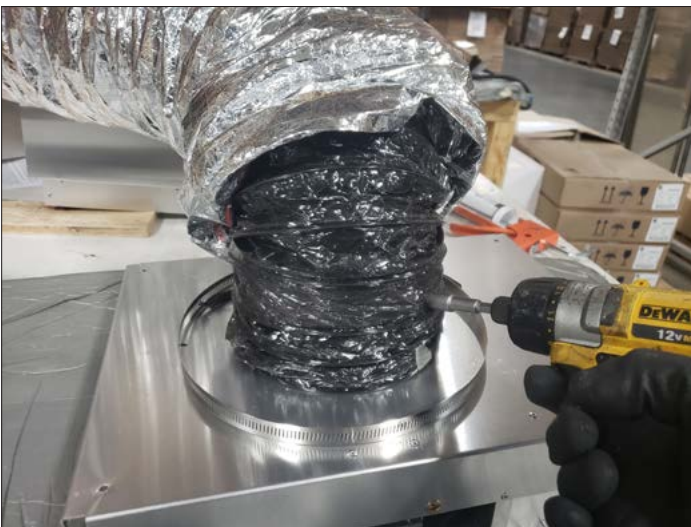
Figure 2.16, Screws in Inner Liner
