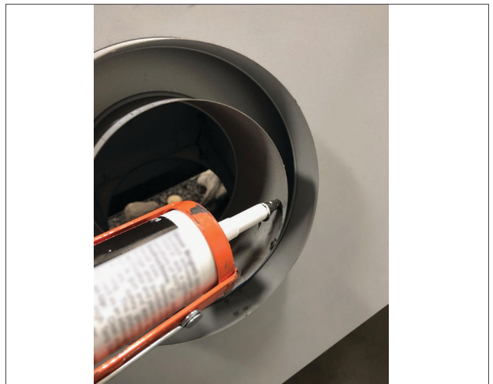
Figure 2.2, Silicone Inner Exhaust on Fireplace
